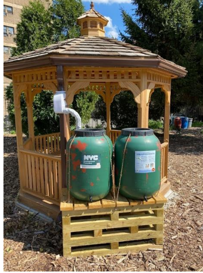
Rainwater harvesting system with rain barrels attached to gutter
